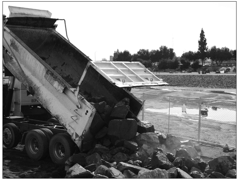
The Orange County Public Works department is beginning a project near the Santa Ana riverbed by Chapman Avenue and the 22 Freeway to help with flood prevention, said Orange County Public Information Officer Carrie Braun.
